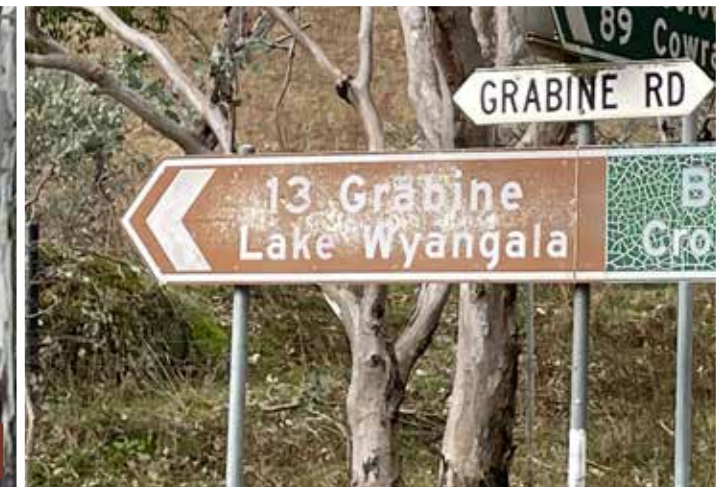
Directional sign faded and in need of replacement
