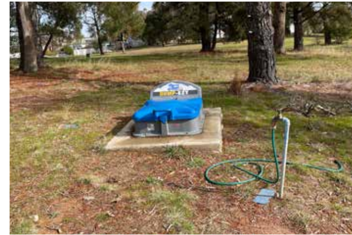
Bigga Recreation Ground RV dump point - directional and positional signage to this location required
