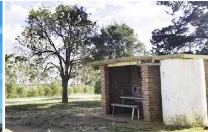
Touts Lookout - basic facilities in need of maintenance or replacement
