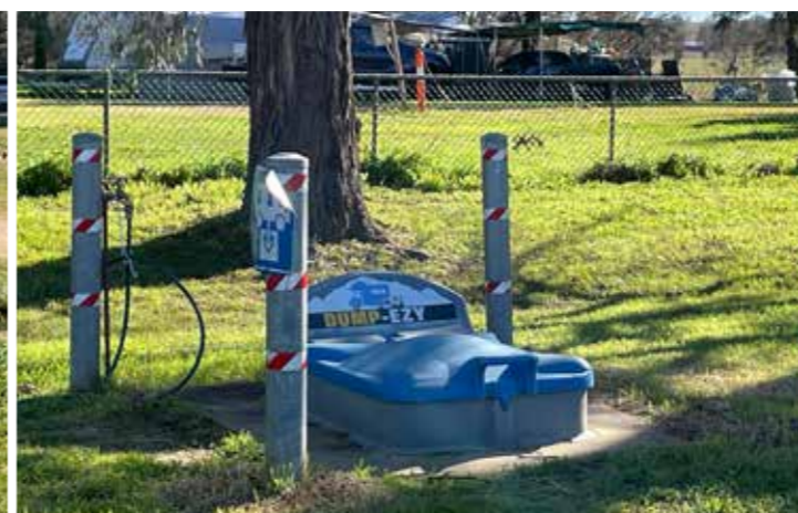
Boorowa RV dump point - directional signage to this location is good but let down by poor positional signing
