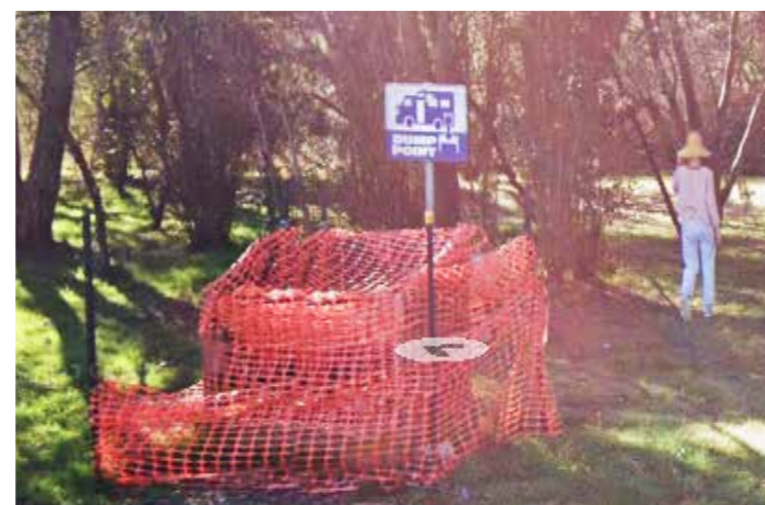
Braidwood - Newly constructed RV Dump Point at Bicentennial Park. Install AS symbol at this dump point
