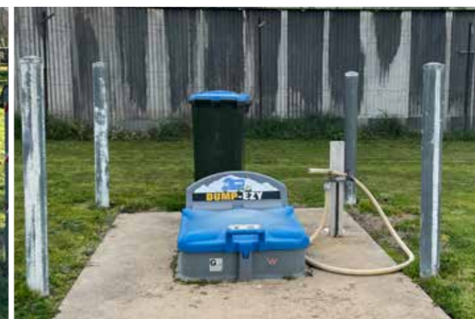
Harden RV dump point - No directional signage from Burley Griffin Way or internally within the showgrounds
