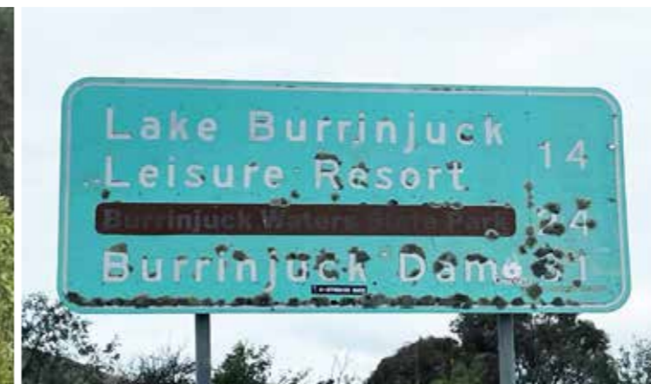
Hume Hwy - Burrinjuck Rd trailhead sign in need of replacement
