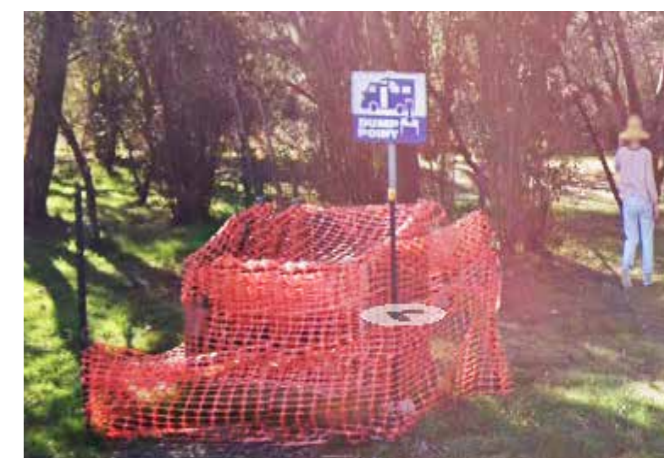
Braidwood - Newly constructed RV Dump Point at Bicentennial Park. Install AS symbol at this dump point
