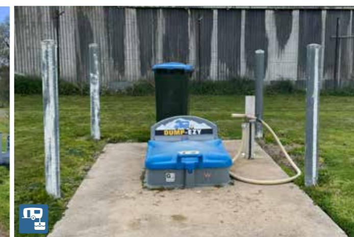
RV dump point - should have positional sign as the facility can be hard to locate especially when there are equestrian events on (horse floats)
