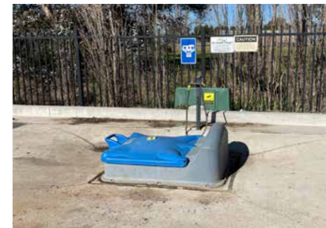
Goulburn - Braidwood Rd RV Dump Point
