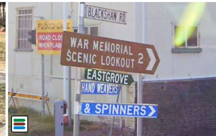
Goulburn - Signage structure at Sloane St/Blackshaw Rd intersection in need of replacement.
